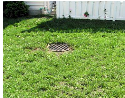
Typical yard drainage unit
