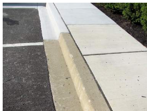
Typical sidewalk and curb and gutter. Note: section of both have been replaced
